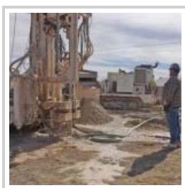
Don McDermott / Pahrump Valley Times – Enlink Geothermal Services developed the earth heat exchange system at PVHS, which is part of a campus expansion project underway.
